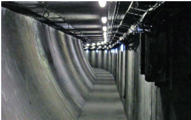
View under the carriageway of the Queensway Tunnel between Liverpool and Birkenhead. Note the curved side of the tunnel. This passageway carries cables and can be used as an escape route if necessary
